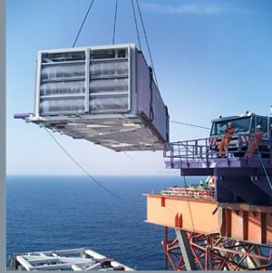
Maintenance, modifications and operations
